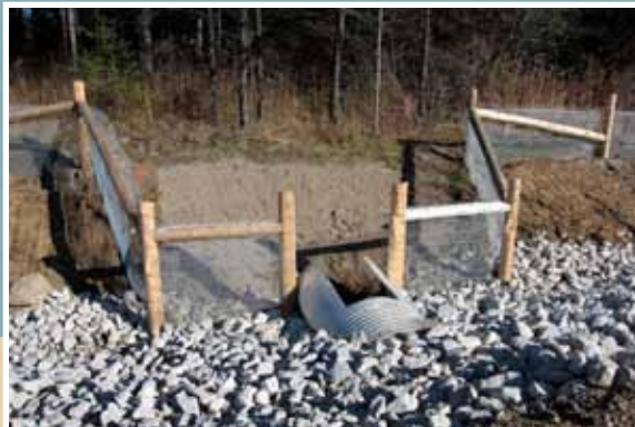
Figure 17 : Installation of a steel culvert and barrier fencing to facilitate turtle movements across Highway 10 near Orangeville. © MTO.
